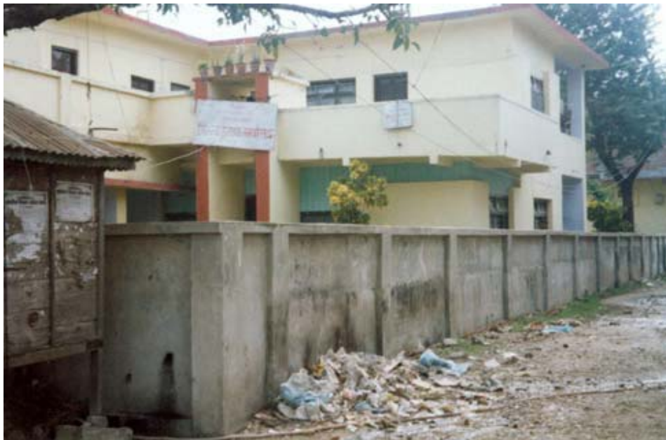
Haphazard Disposal of Waste in Front of District Postal Office
